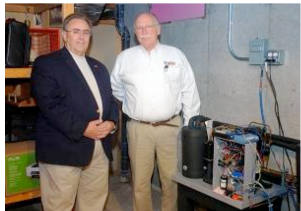
Larry Tracey and Sam Johnston II, of Terraclime Geothermal , pose next to geothermal unit in Tracey's basement in Enfield on Monday February 8, 2010. (Leslloyd F. Alleyne/ Journal Inquirer).
